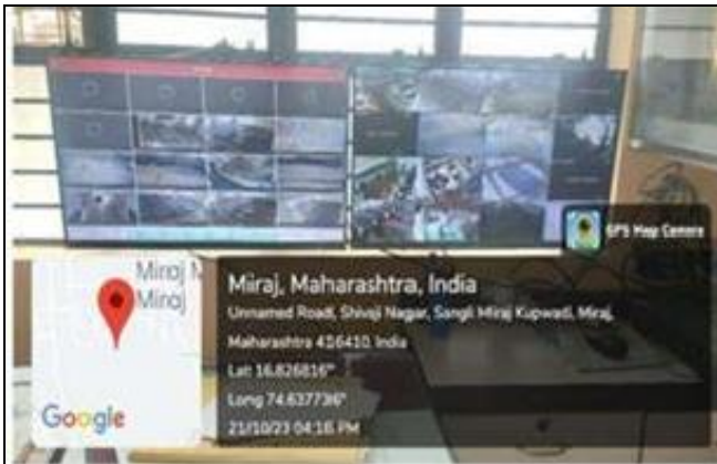
CCTV Camera Recording Control Room
