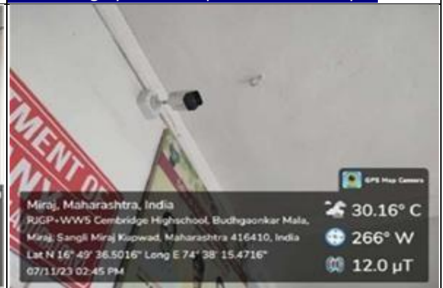
CCTV Camera at Microbiology Department
