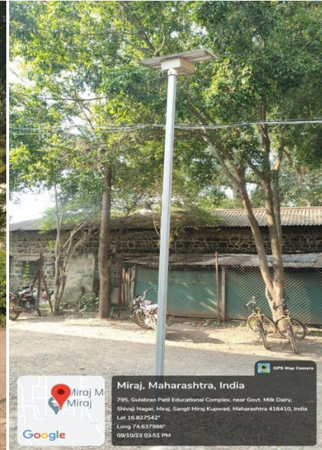
Solar Street Light
