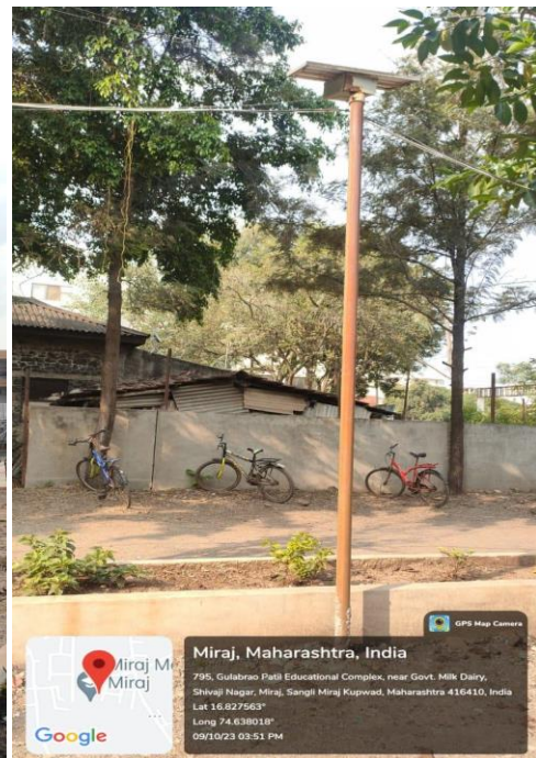
Solar Street Light
