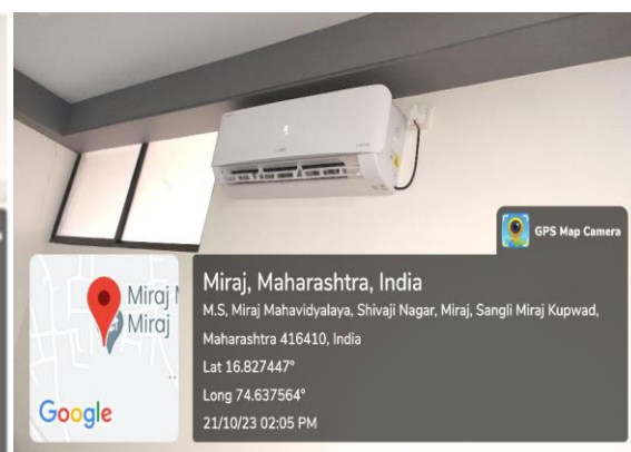
Power Efficient AC –IQAC/NAAC Room
