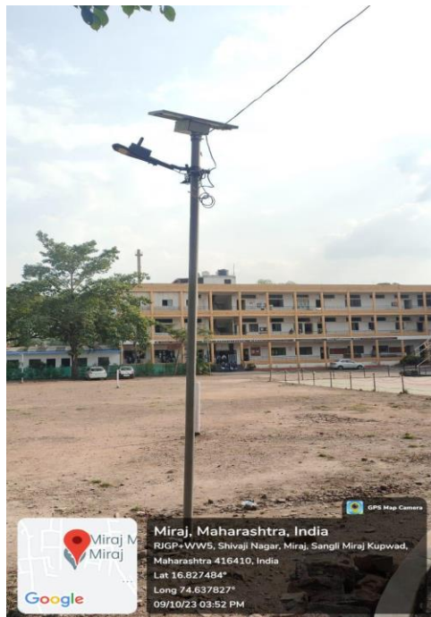
Solar Street Light
