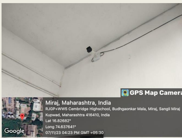
CCTV Camera at Microbiology Dept
