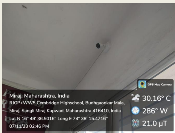
CCTV Camera at Chemistry Department
