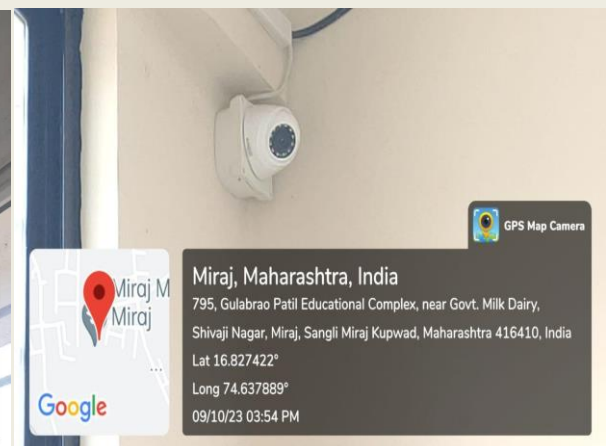
CCTV Camera at Consumer Store
